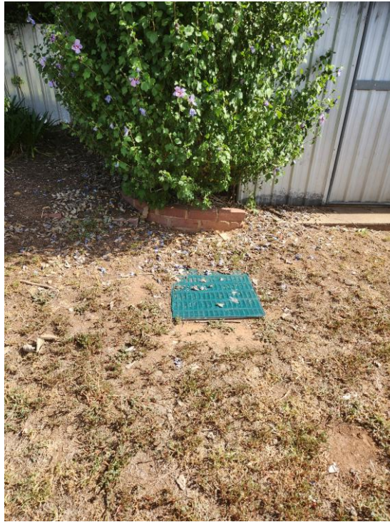
Existing stormwater drainage pit '2' in rear yard, adjacent north-east corner of existing garden shed. This pit forms part of the council drainage main pipe
