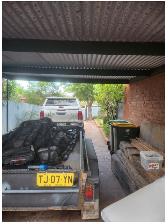
Existing carport area to replaced with new, longer carport to allow more adequate required secure shelter for vehicles, trailers etc.
