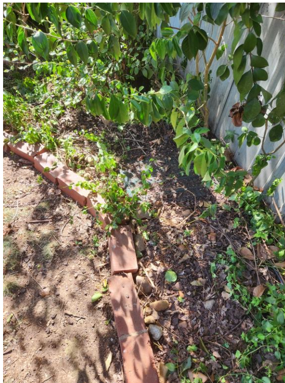
Existing stormwater drainage pit '1' in rear yard, within north garden bed This pit forms part of the council drainage main pipe
